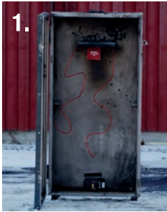
1. A lithium battery was placed at the bottom of the cabinet and the MAUS unit/units were placed at the top.
